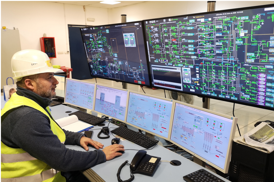
FactoryTalk View Enterprise SCADA operator station
